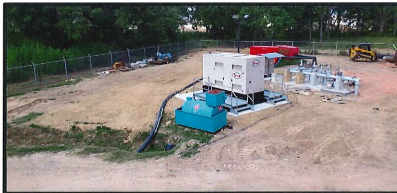
Lift Station Site
