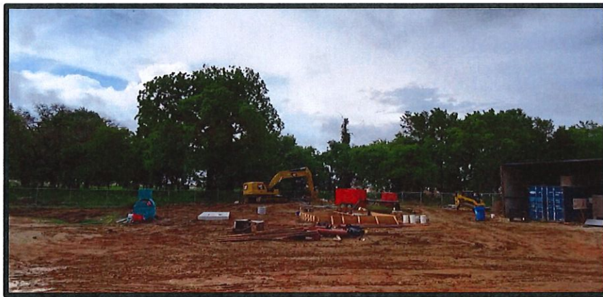
Lift Station Site
