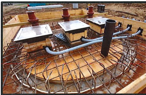
Lift Station No. 1 Wet Well
