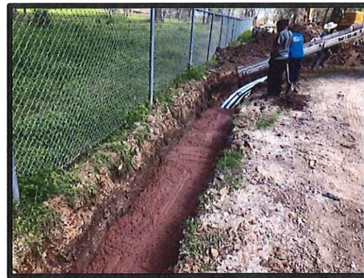
Electrical Duct Bank
