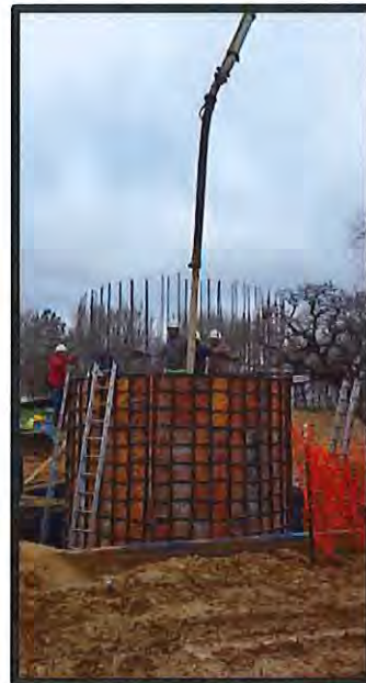
Lift Station No. 1 Wet Well
