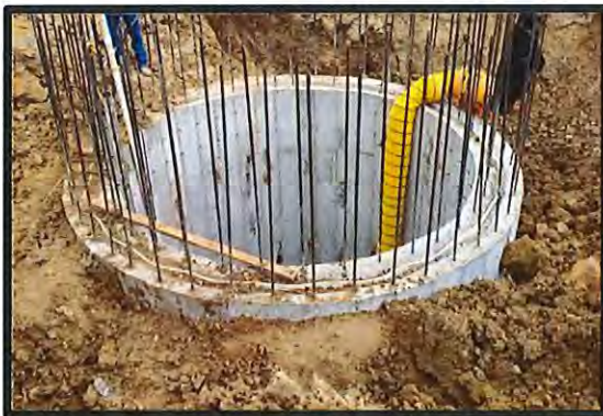
Lift Station No. 1 Wet Well
