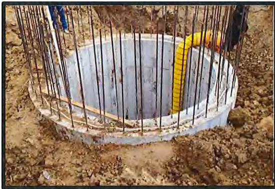
Lift Station No. 1 Wet Well
