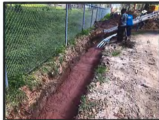
Electrical Duct Bank
