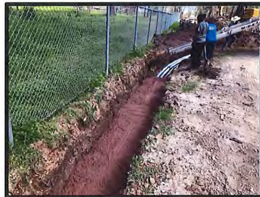
Electrical Duct Bank
