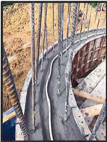
Lift Station No. 1 Wet Well
