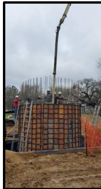
Lift Station No. 1 Wet Well
