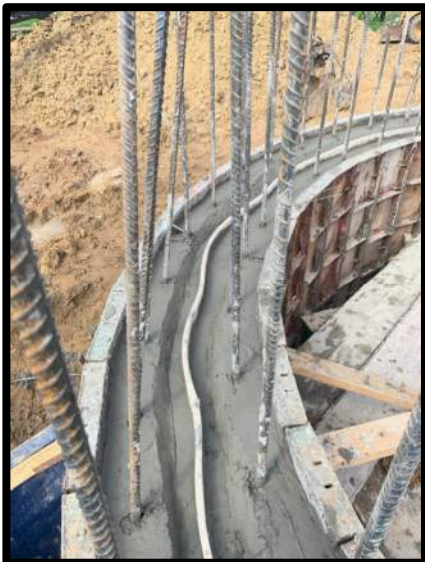
Lift Station No. 1 Wet Well
