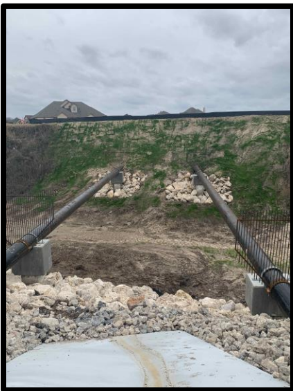
Water and Sanitary Sewer Lines
