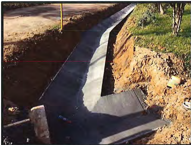
Roadside ditch along MLK Drive
