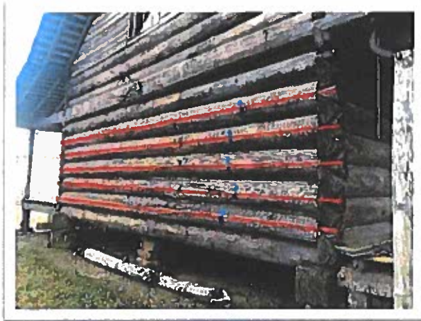
North wall. Red lines indicate logs to be replaced
