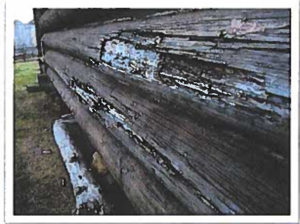
Closeup of the rot
