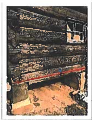
Red line indicates log to be replaced
