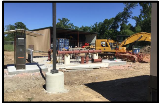
Lift Station Site
