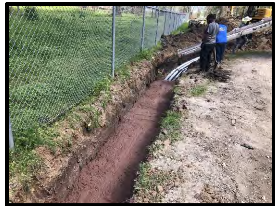
Electrical Duct Bank
