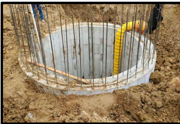
Lift Station No. 1 Wet Well
