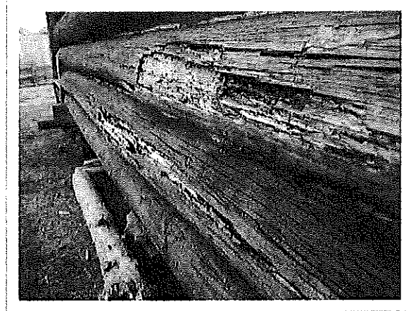
Closeup of the rot
