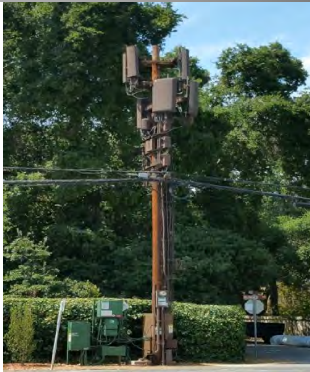
Example of a cluttered small cell install
