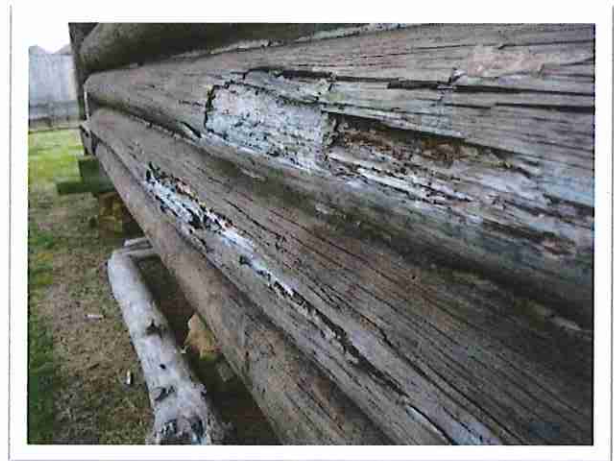
Closeup of the rot
