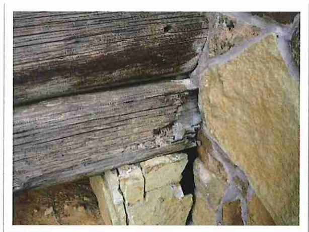
Closeup of the rot close to the chimney
